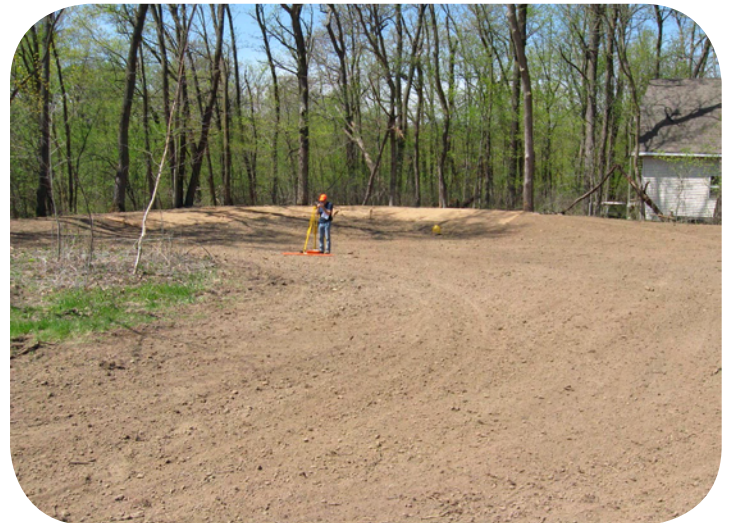
After: A berm at the back corner of the field allows water to temporarily pond before flowing out more slowly through the outlet structure into the gully.
