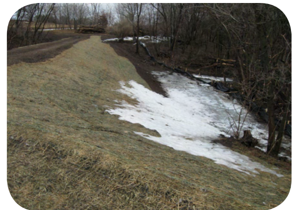
After: A berm backs up the runoff water, which outlets more slowly to the gully.
