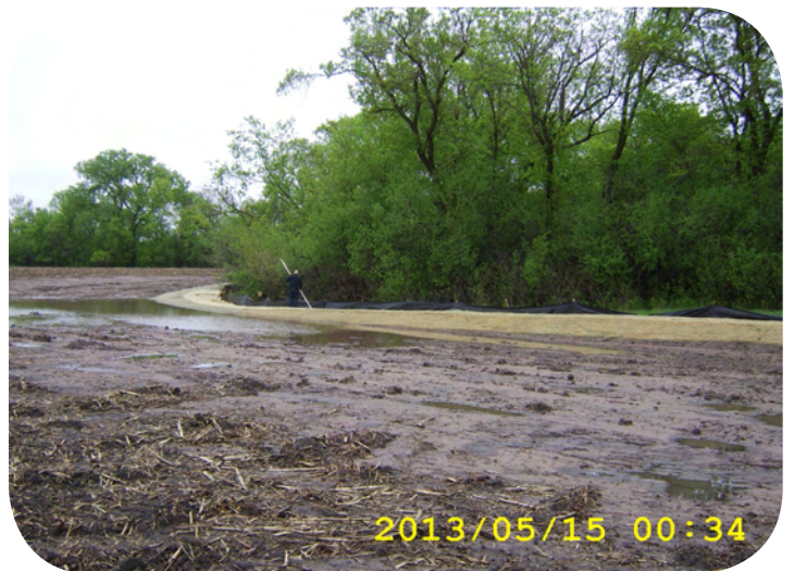
After: A berm along the edge of the field allows water to temporarily pond before flowing out more slowly through an outlet structure into the woods.
