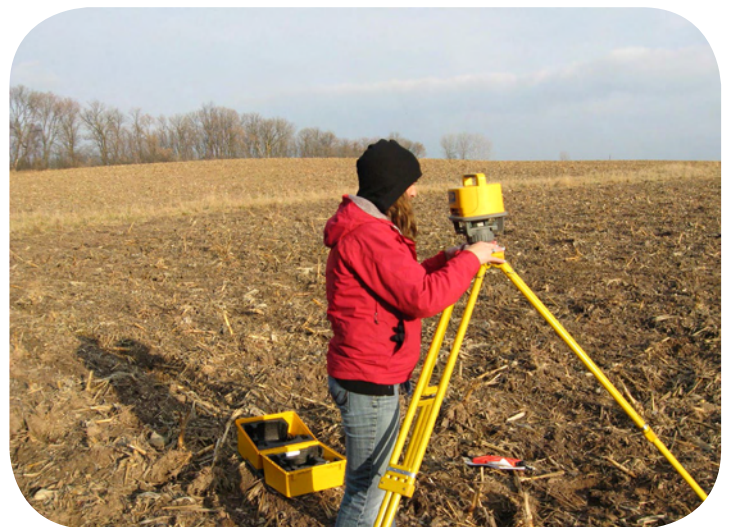
Above: WCD employee Tara Kline surveys the field where the sediment basin will be built.
