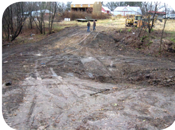
Before: Runoff was creating a gully and erosion.
